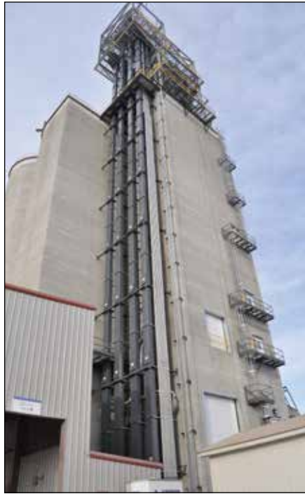
Ground-level view of four 20,000-bph Schlager legs mounted outside of the slip.
