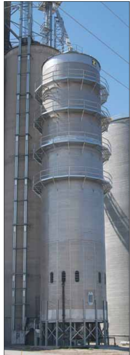
New 7,000-bph Zimmerman natural gas grain dryer installed at Sedan.
