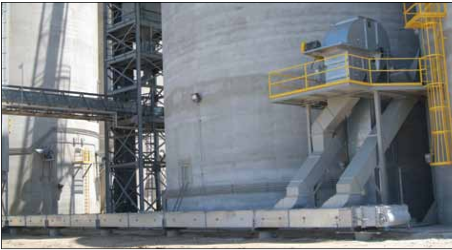
New tanks at Aurora West empty via Schlagel jump legs onto a Hi-Roller enclosed belt conveyor running back to existing grain handling equipment.
