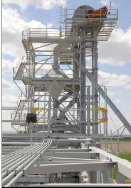
Equipment atop the LeMar support tower includes a J & D 20,000-bph gravity screener and Schlagel double distributor.
