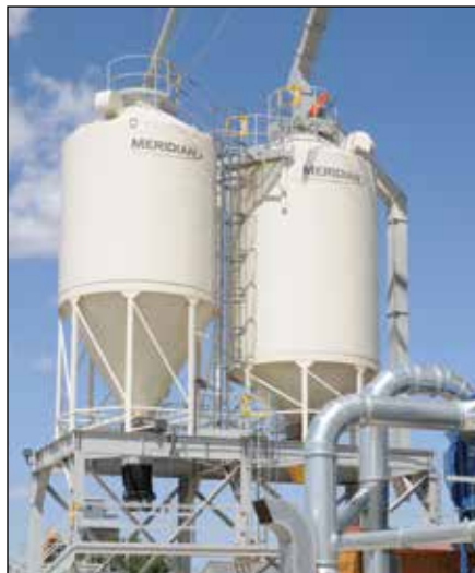
Two Meridian welded steel tanks handle corn and screenings, respectively.
