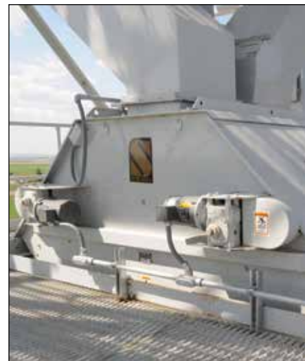
Seven-duct Schlagel SwingSet distributor can send grain to storage, dryer, or truck loadout.
