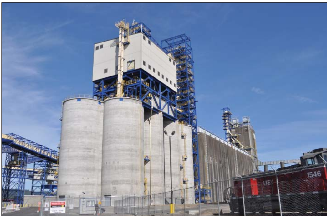
Slipform concrete shipping bins in foreground hold nearly 500,000 bushels. New cleaning house is mounted directly atop the shipping bins. Ground level photos by Ed Zdrojewski.
