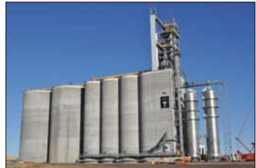
Ground-level view of the new Gavilon elevator nearing completion in early November, one week after a ribbon-cutting open house and already receiving grain. Ground-level photos by Ed Zdrojewski.
