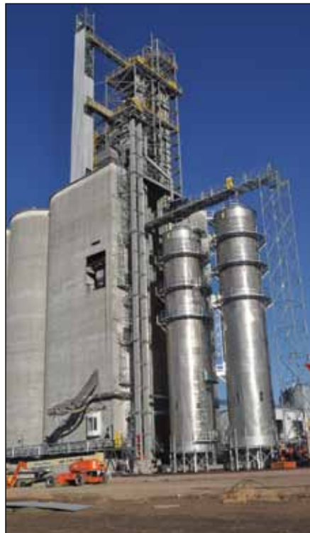
Grain receiving and rail loadout tower shown with twin Zimmerman 4,700-bph tower dryers.
