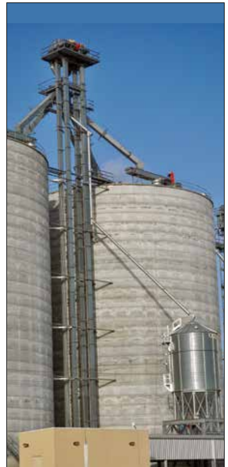
A pair of 20,000-bph Schlager receiving legs lift grain up to a six-hole Schlager swing-type distributor. Also visible is a 5,000-bushel Brock surge tank for loading trucks.
