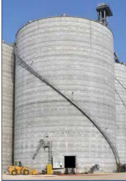
Hoffmann Inc. equipped one of the four 650,000-bushel silos with a spiral staircase for easier climbing. All four silos have Bobcat doors as shown.
