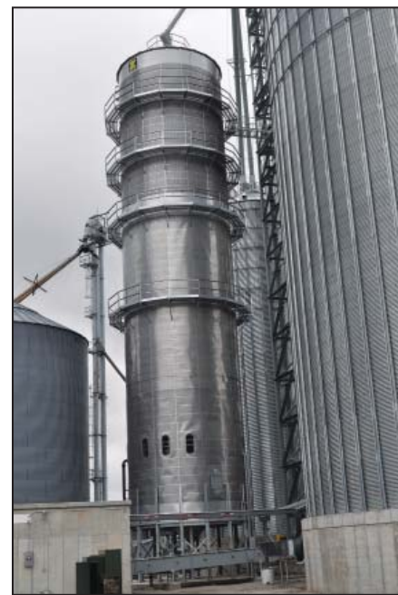
A 7,000-bph Zimmerman Dryer was installed in 2012.
