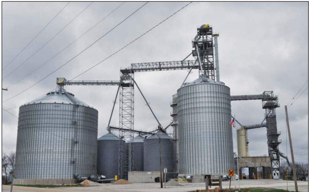
Alliance Coop upgraded its Anchor, IL facility in 2011-13 with four steel tanks, four bucket elevators, a dryer, and two dump pits. Photos by Ed Zdrojewski.
