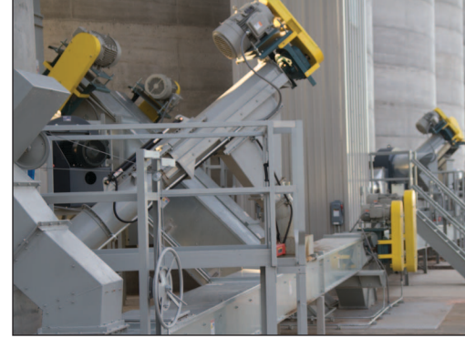
The hopper bottom concrete tanks empty via gravity or via an auger onto a 10,000-bph Intersystems drag conveyor.
