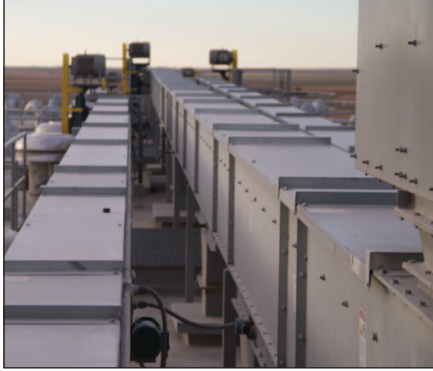
The jumpform tanks are filled via overhead 20,000-bph Intersystems drag conveyors.
