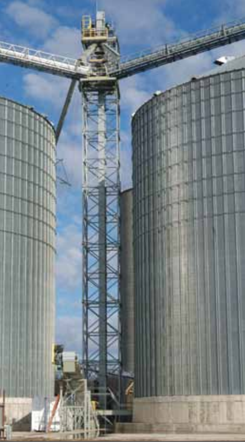
New 20,000-bph receiving leg accepts grain from the newest of the facility's five receiving pits.
