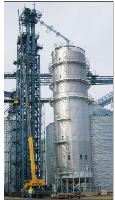
New 10,000-bph Zimmerman tower dryer, adjacent to a pair of 40,000-bph legs, one of which was extended upward by 40 feet, in order to elevator grain high enough to reach new storage.
