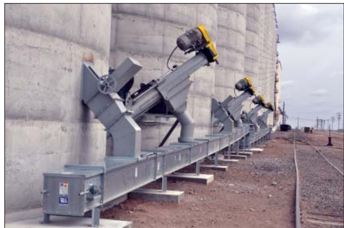
Tank cone bottoms are emptied via augers onto a 10,000-bph drag conveyor running back to existing equipment.
