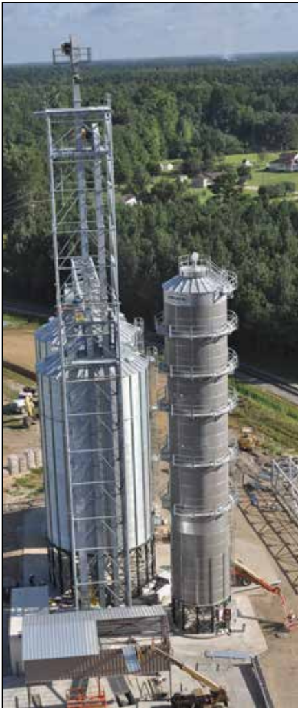
New steel annex includes a pair of 55,000-bushel Brock steel hopper tanks, 4,700-bph Brock tower dryer, Union Iron legs, and Union Iron support tower.
