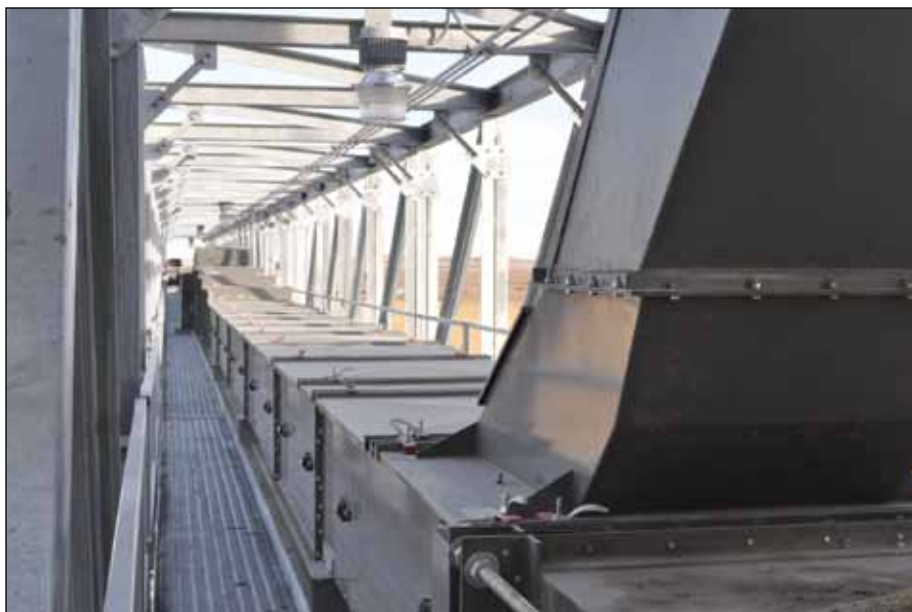
A series of 32,000-bph Hi Roller enclosed belt conveyors, encased in a 9-foot-wide Warrior box truss, carry grain from the distributor out to upright storage or a temporary storage pile.
