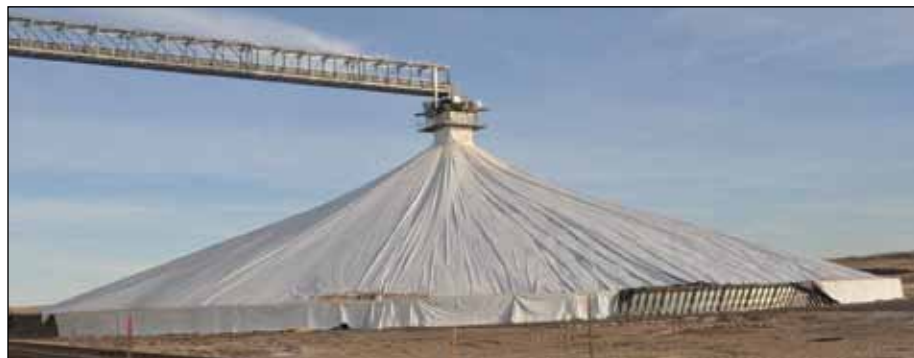
New 2-million-bushel LeMar temporary storage pile features six-foot perforated steel sidewalls, compacted fly ash floor, and aerated center-fill tower system.
